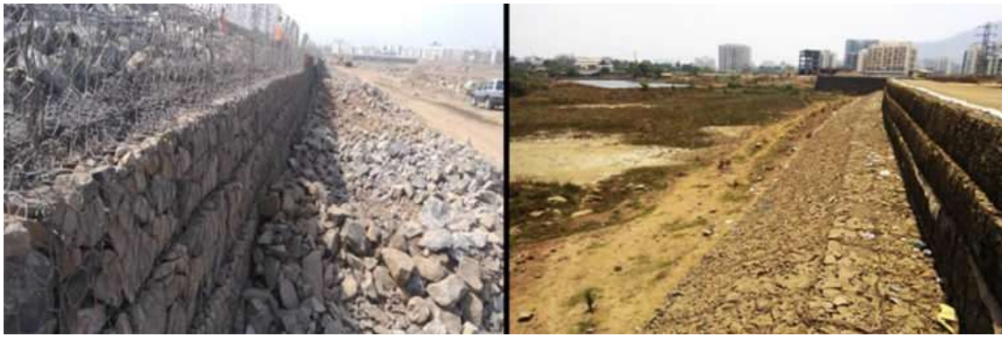
The finished gabion – reinforced soil wall. The airport is expected to open in 2023.
