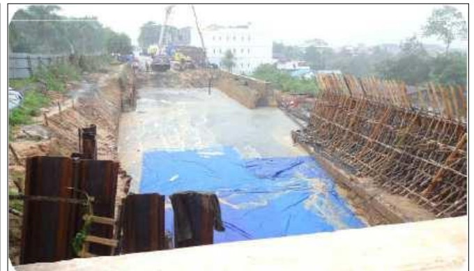
During heavy rains
