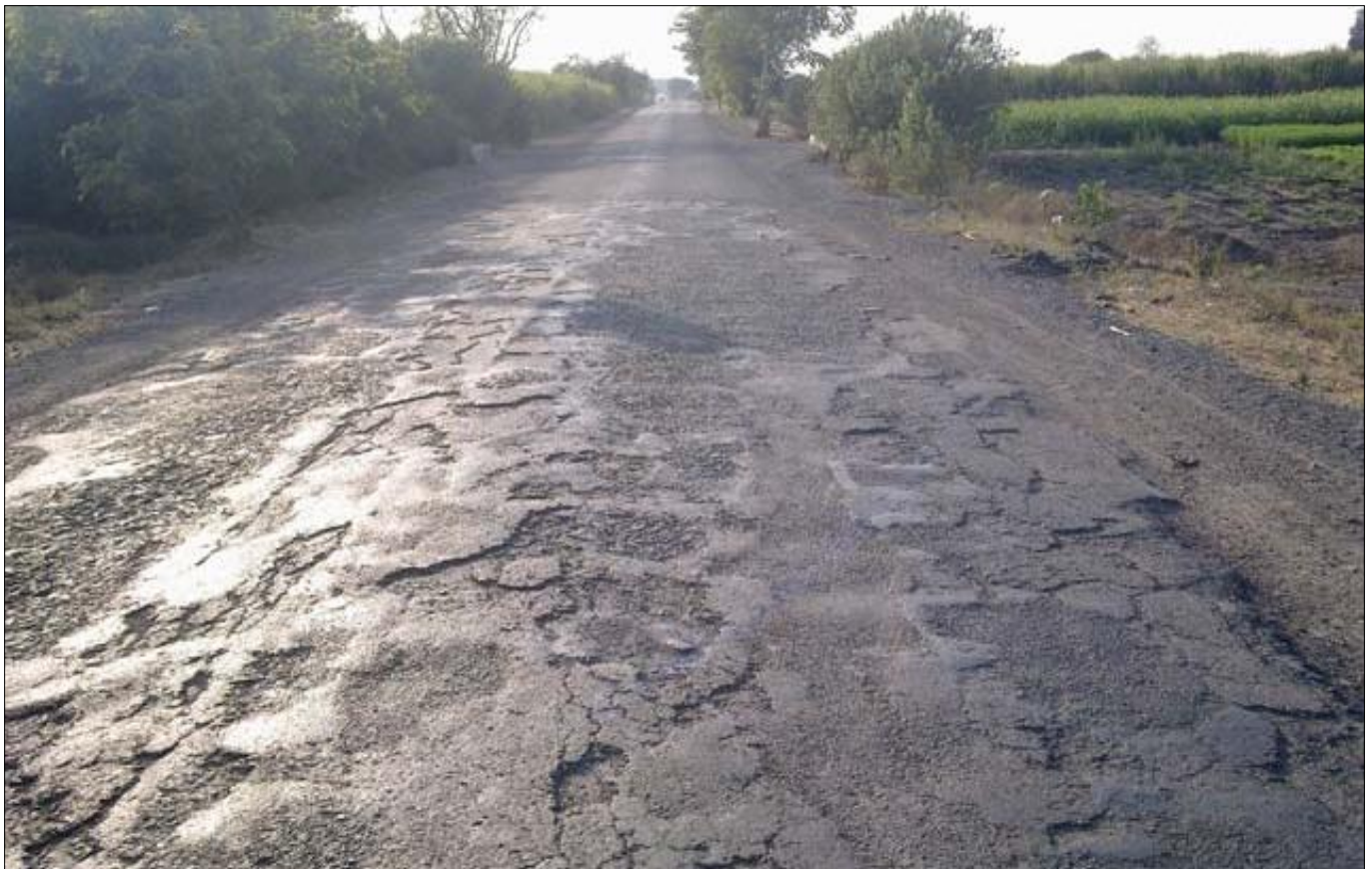
Distressed Pavement with Cracks
