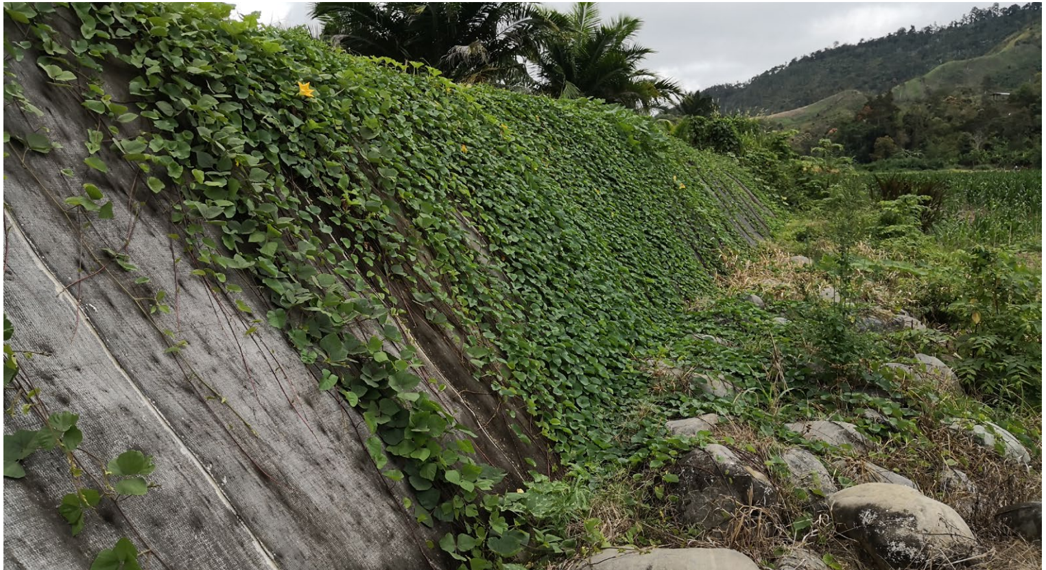
Vegetation growth at the toe and crest of the bank installaton, CCX-M™ is still performing as expected
