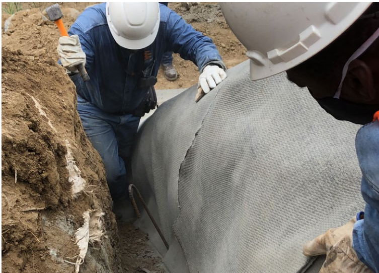
The edge of the CCX-M™ was pegged at the base of the anchor trench
