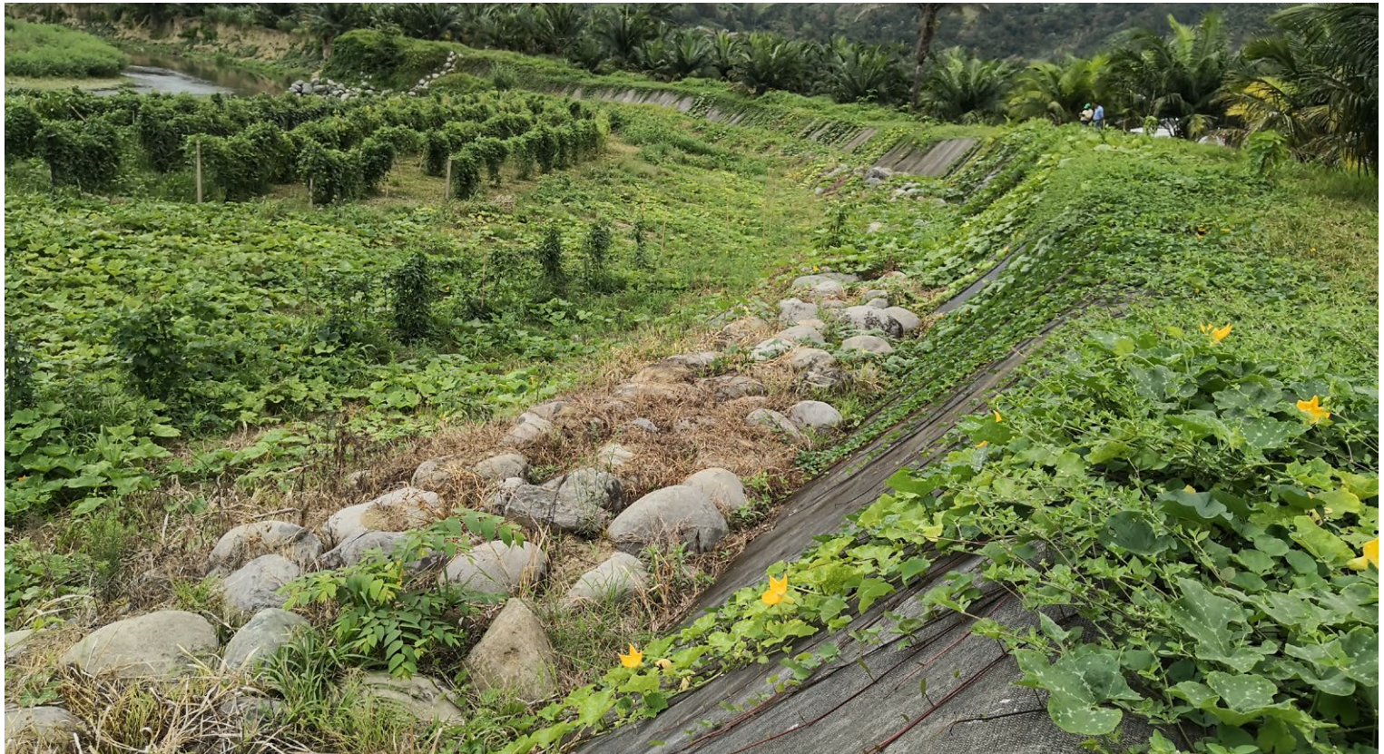
Vegetation growth at the toe and crest of the bank installaton, CCX-M™ is still performing as expected
