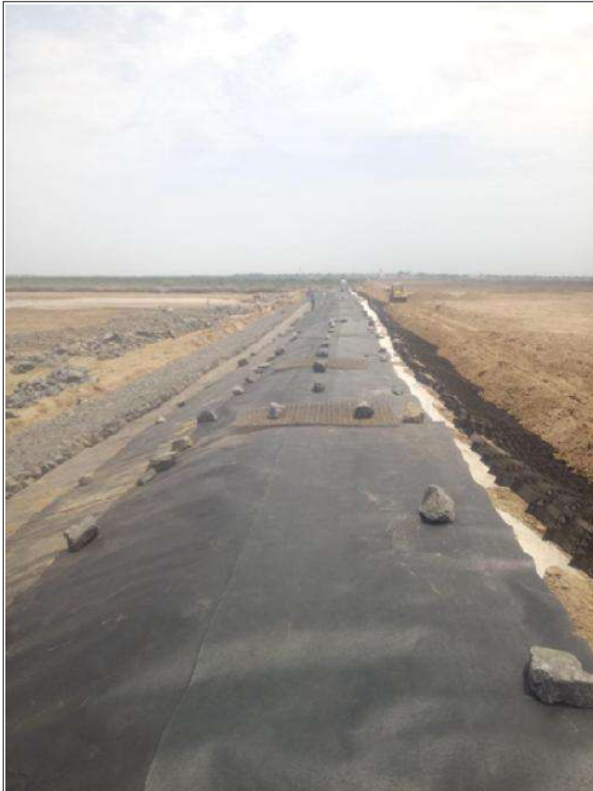
Geomembrane & Nonwoven geotextile layer is laid and Gabion Mattress installation in progress
