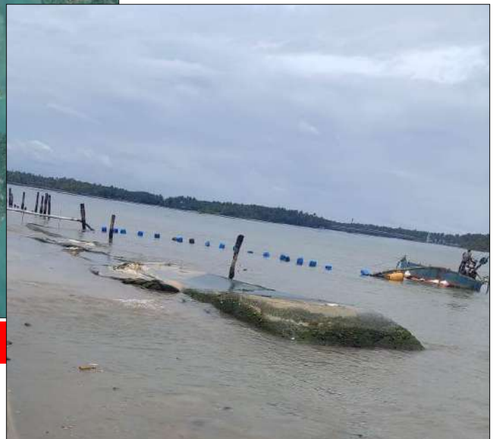
Damaged existing Geotextile Tubes
