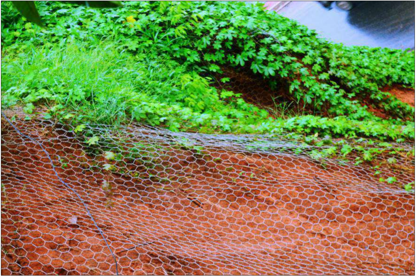
Structure after 7 years
