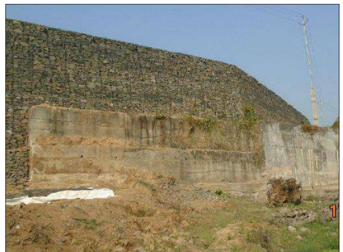
Reinforced Soil Wall with Gabion facia
