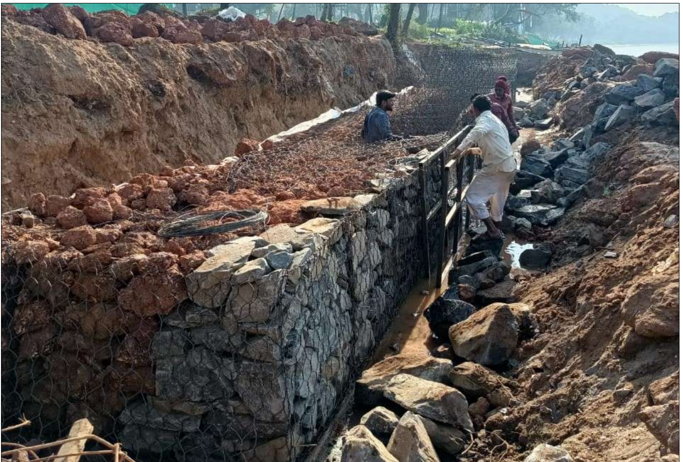
During Construction Photographs. Back side filling of units done with locally available lateritic boulders
