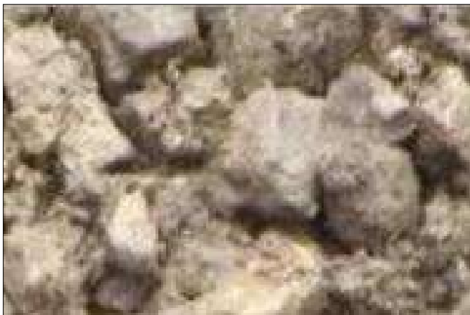
Photo 3 : Ballast penetration in to the subgrade
