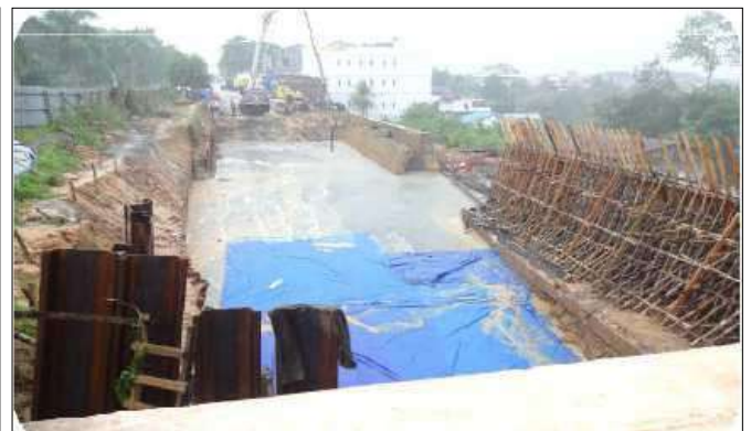
During heavy rains
