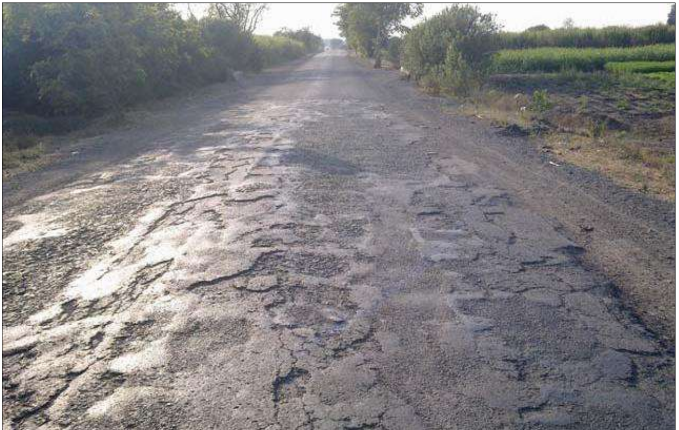
Distressed Pavement with Cracks
