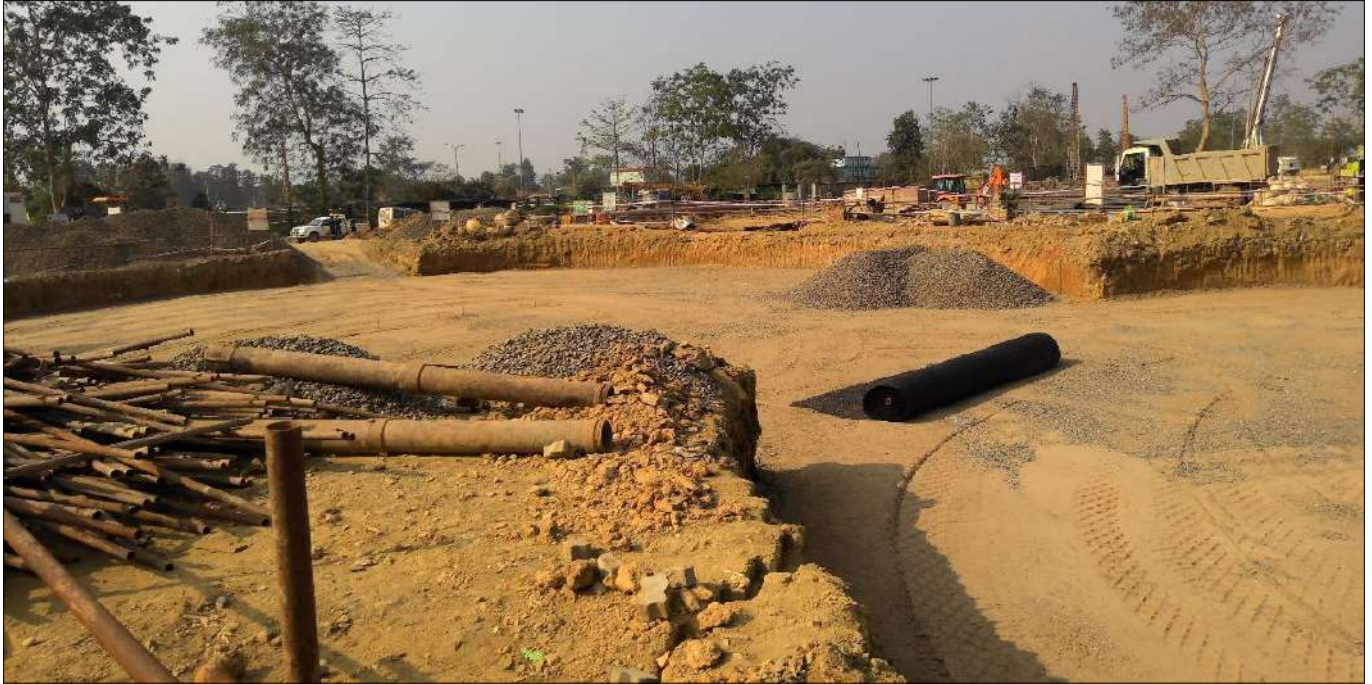
Photo 1 : Prepared Surface for Laying Geogrid & Rolls of Geogrids are ready to be laid
