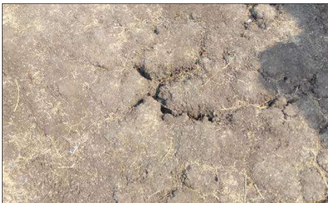
Shrinkage cracks in the existing subgrade soil
