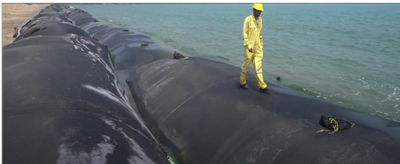
After complete laying Geotextile Tube in base layer and in middle layer (3+2 )
