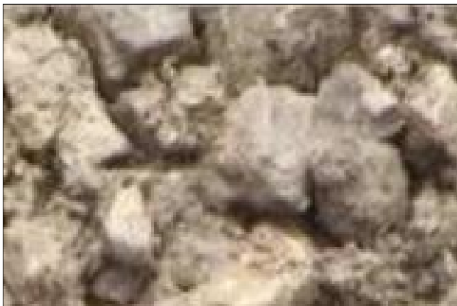
Photo 3 : Ballast penetration in to the subgrade
