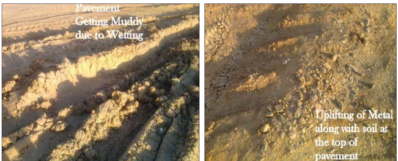
Fig 1 : Existing Deformed Pavement
