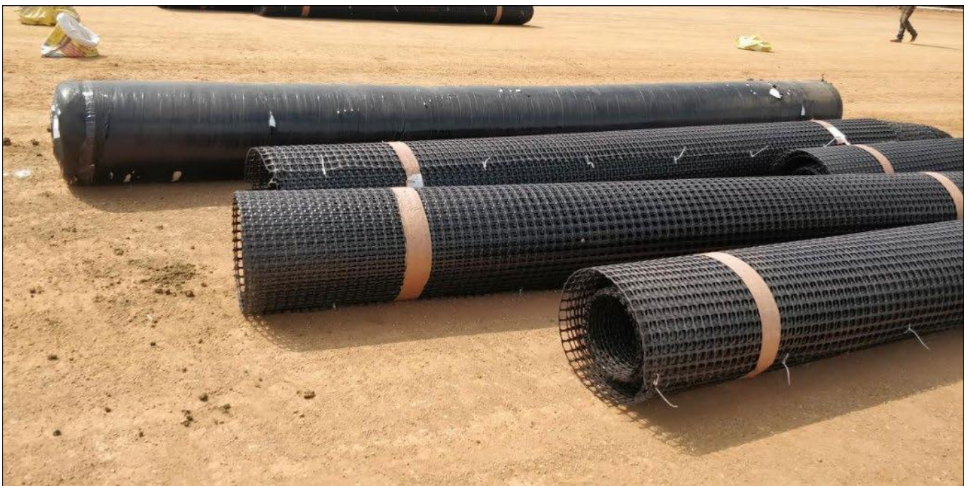
Rolls of Techgrid PP biaxial Geogrid and Techgeo Non-Woven Geotextile ready to be laid
