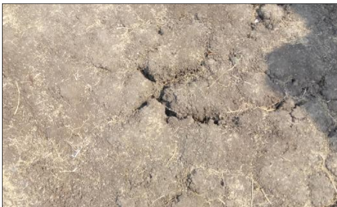
Shrinkage cracks in the existing subgrade soil
