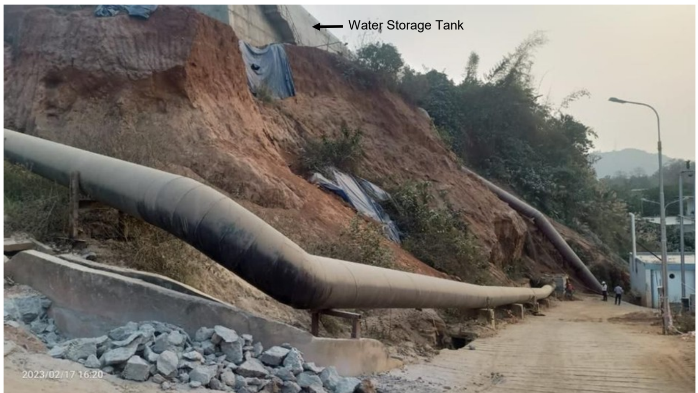
Photo 1 : View of Exposed Slope experiencing erosion and cavity due to loose soil detachment
