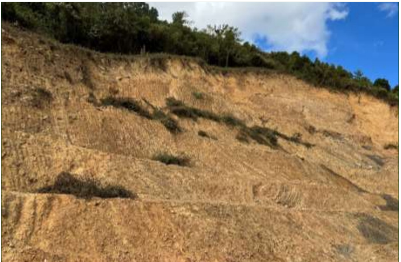
Photo 1 : Exposed Hill-side cut slope with overburden strata over weathered rock along package 8
