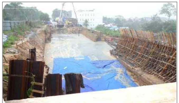
During heavy rains
