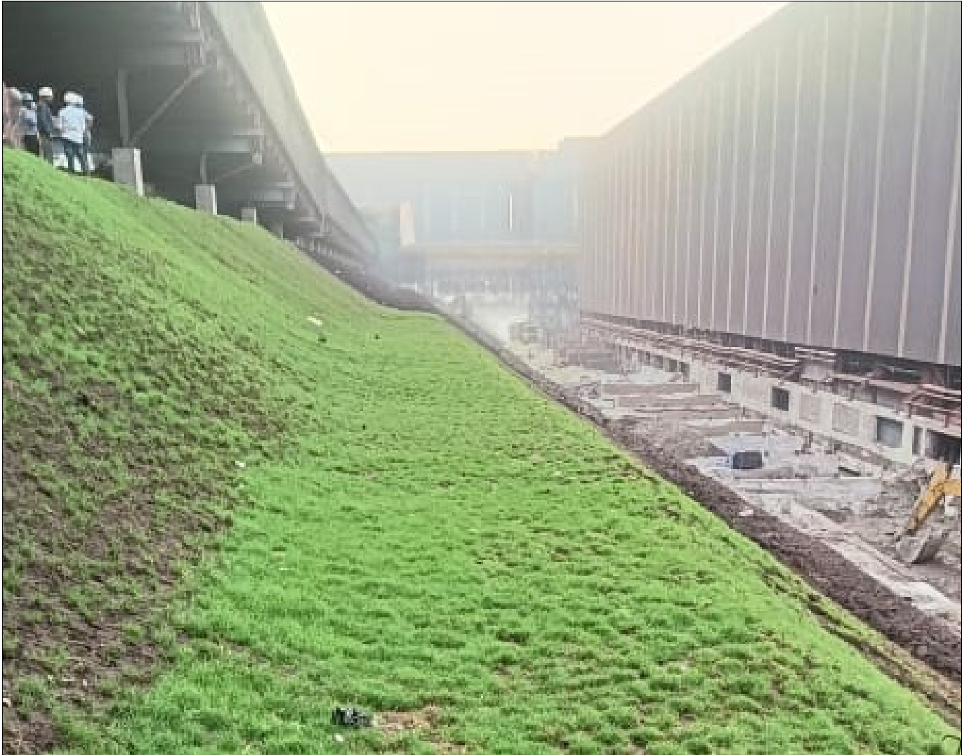
Photo 7 : Slope Stabilized with Growing Vegetation
