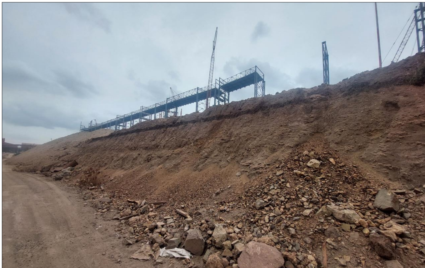
Photo 1 : Pre-Construction Site Condition : Unstable Slope
