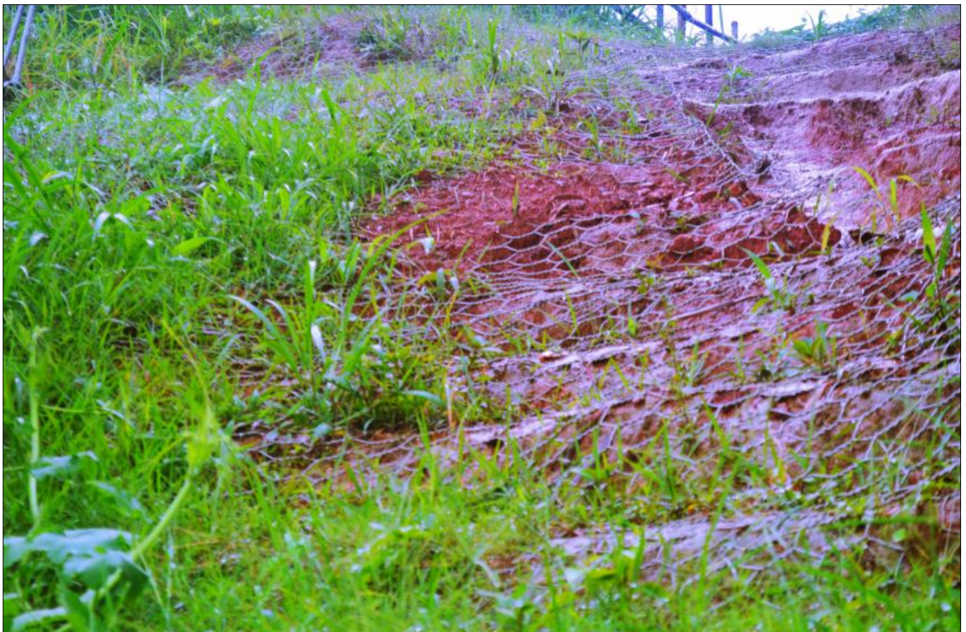
Top of Slope after Vegetation has grown
