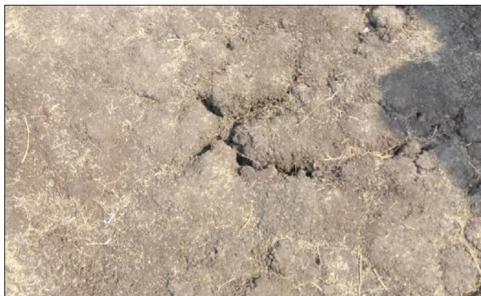
Shrinkage cracks in the existing subgrade soil
