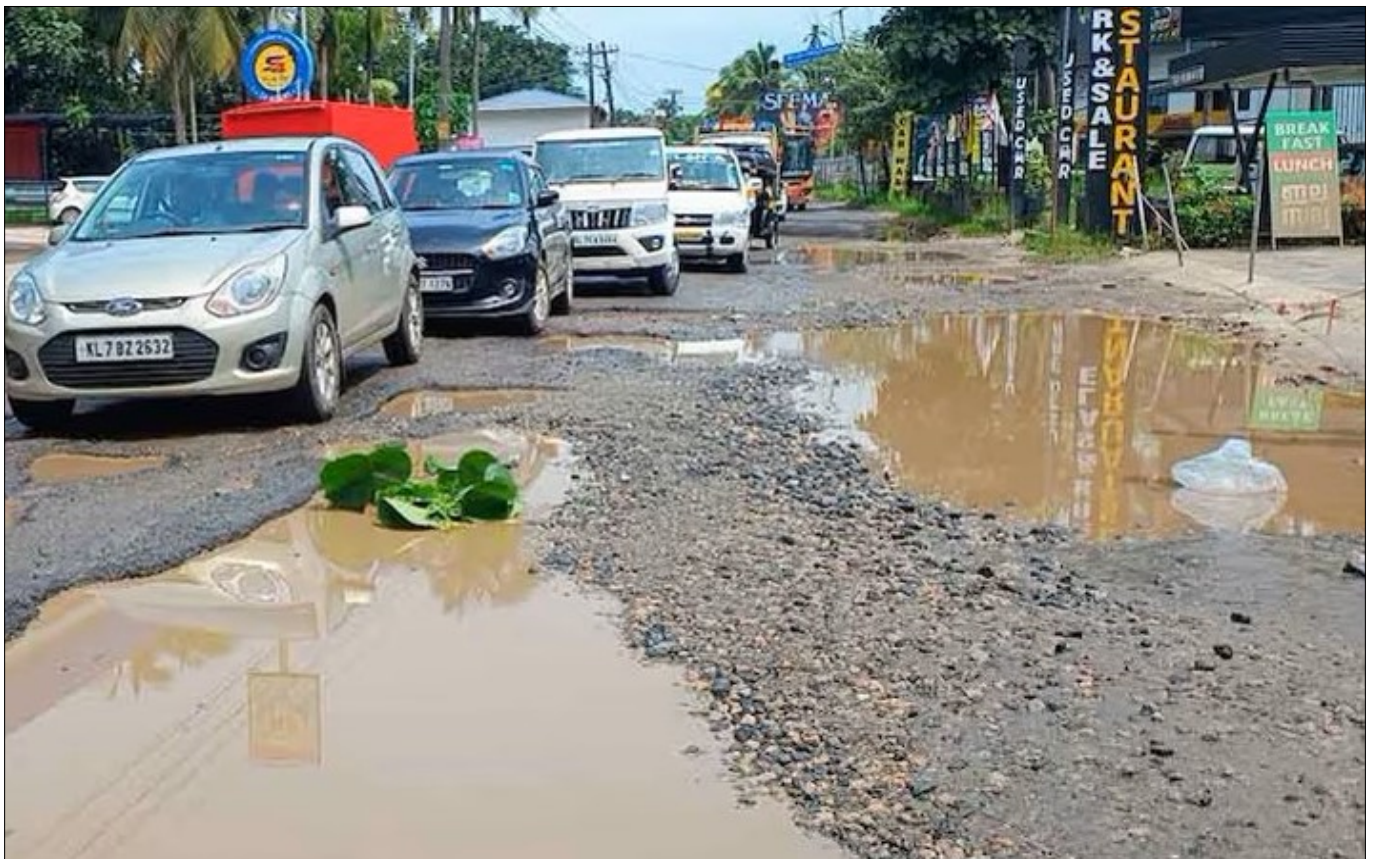
Photo 1 : Damaged Road and Waterlogging on Kecheri Bypass
