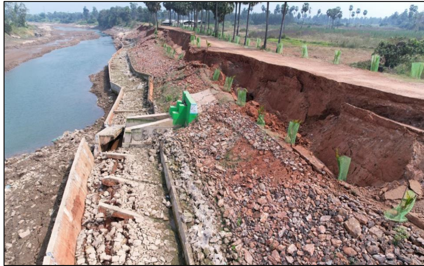
Figure 1: Damaged left side river bank on the Sharda River as of 29 th January 2023
