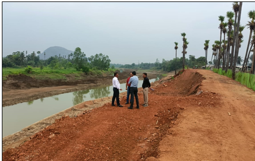
Figure 2: Site Inspection by Authorities of the Damaged left side river bank on the Sharda River as of 18 th Feb 2023
