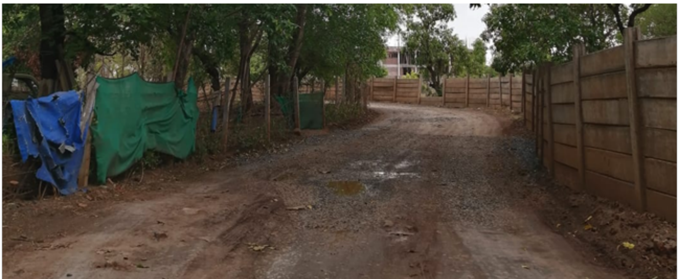
Photo 1 : Initial Condition of the Road
