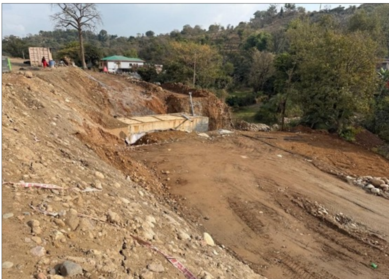
Photo 2 : Pre-Construction Site Condition : Unstable Slope
