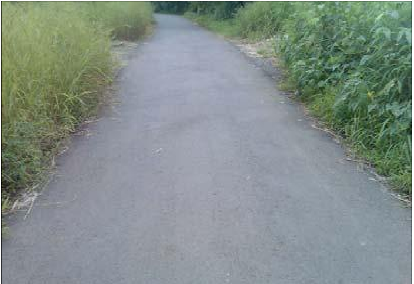
Road Condition after 12 Months (Including Monsoon)
